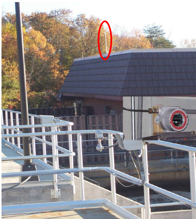
Base Radio Gateway mounted inside control room for ready access and integration with control system I/O
