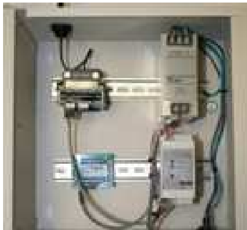
Base Radio Gateway DIN rail mounted with power supply and output module having 4 Analog signals and 8 Switches
