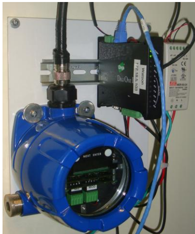
AWS Base Radio Installed @ the Gateway in the Pump Station
